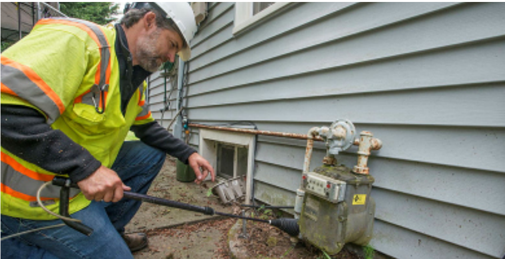
6 A PSE technician checking for gas leaks.
