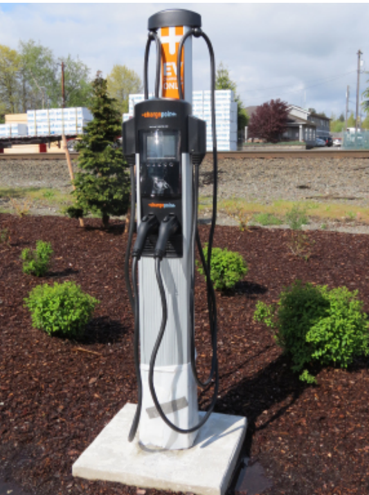
An electric vehicle (EV) charger at the Civic Center.
