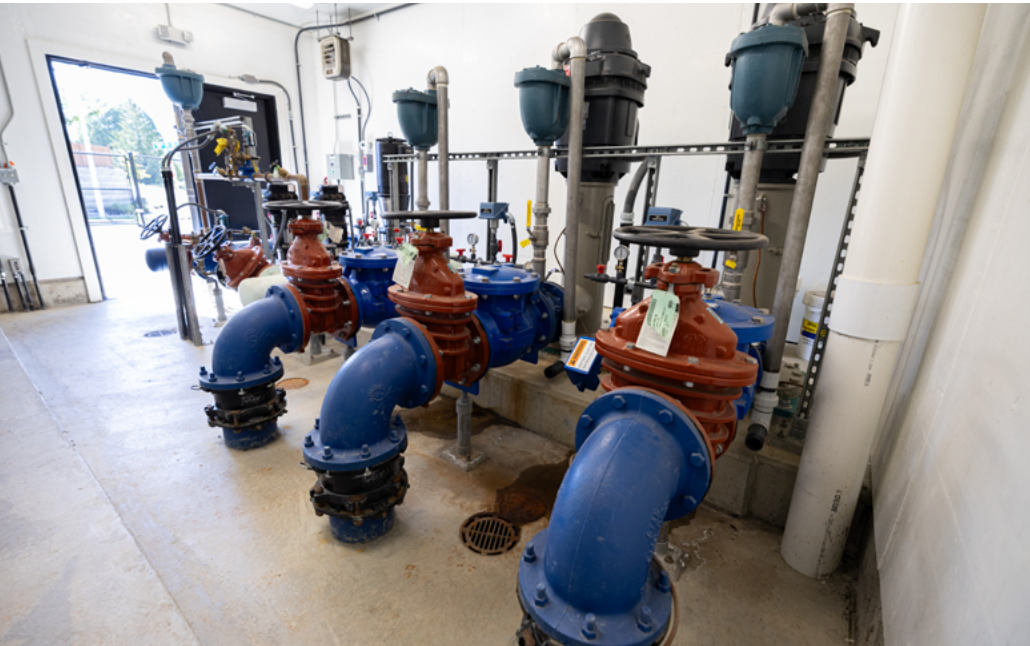
The 560 Zone Booster Pump Station enhances the water pressure and flow in the City’s water distribution system.
