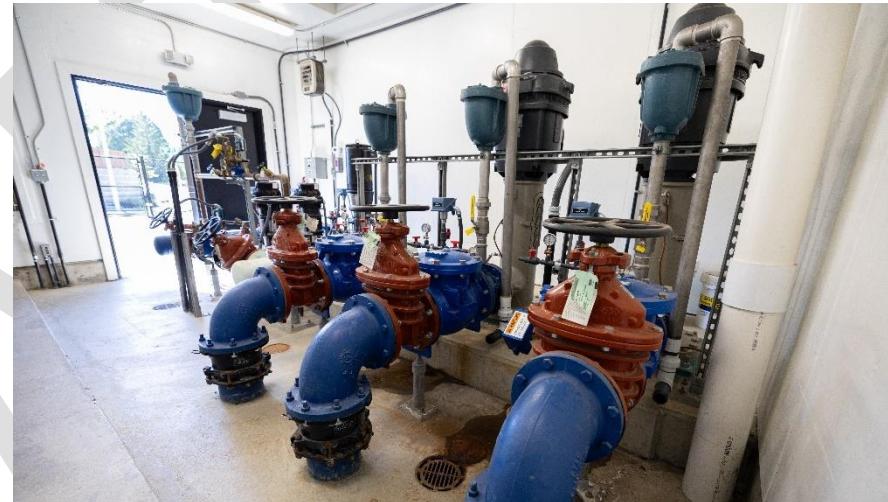
Image 2 The 560 Zone Booster Pump Station enhances the water pressure and flow in the City's water distribution system.
