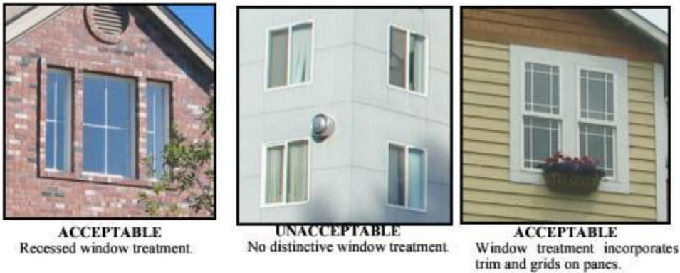
Figure 11 – Acceptable and unacceptable window treatments.
