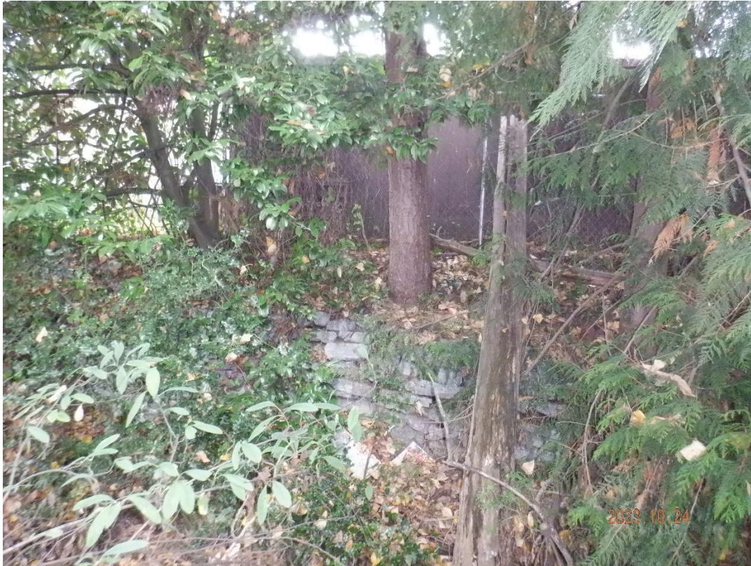
Problematic Douglas fir tree at top of block retaining wall, behind 14405 Timberbrook Drive
